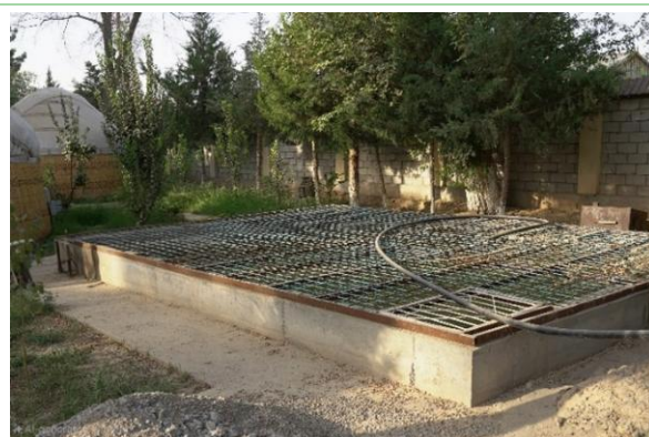
Covered collection/storage structure supporting dry-period irrigation.
