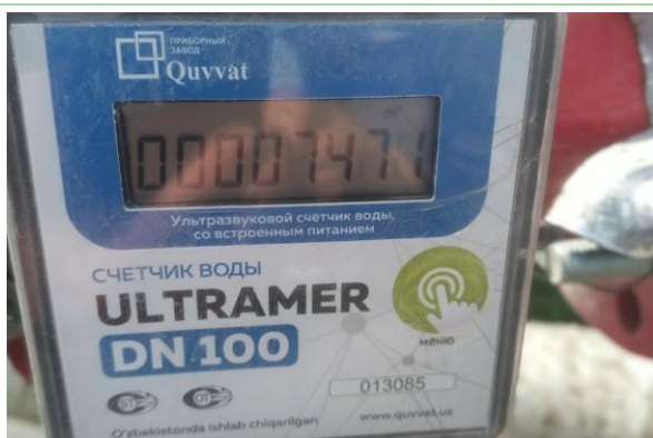
Meter used to record and control water consumption.
