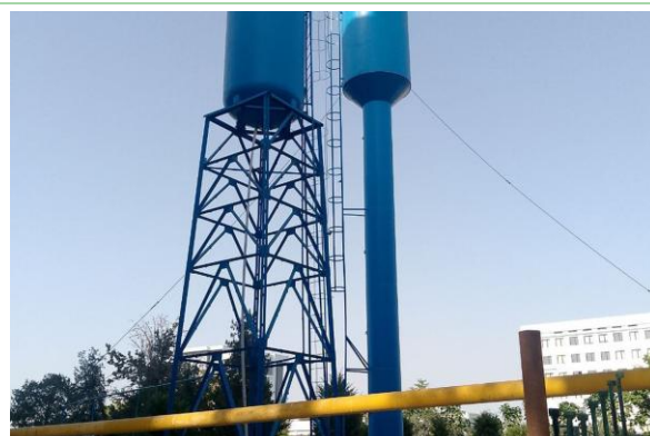
Campus water-storage and distribution infrastructure.
