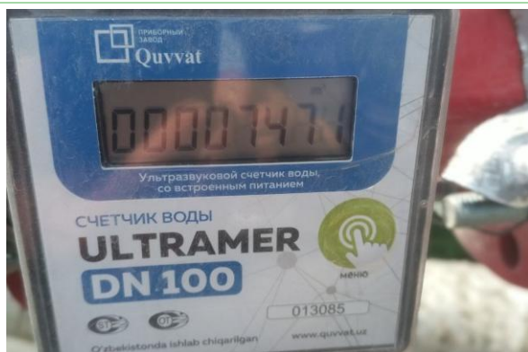
Water meter supporting consumption control.
